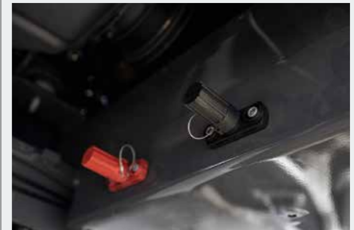
• External battery terminals
